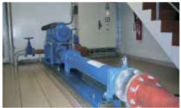
Pump with control box
