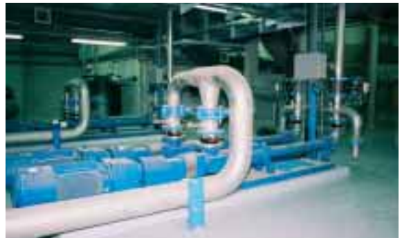
Filter Press Feeding with 2 Moineau Pumps
